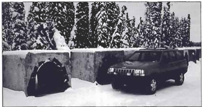
Swamp weights for 48-in. pipeline are stored along a pipeline R.O.W. One weight will control the buoyancy of only 5 m of 48-in. pipeline (Fig. 5).
