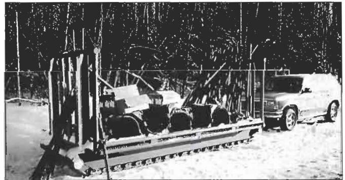
This sled contains enough screw-anchor assemblies to control the buoyancy of 800 m of 20-in. pipeline (Fig. 6).
